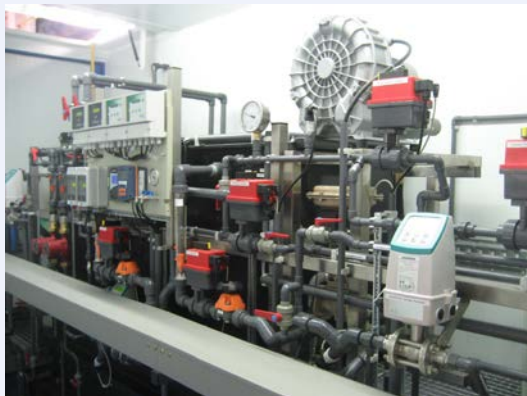
Pilot plant Membrane Bioreactor (MBR)
