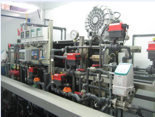
Pilot plant Membrane Bioreactor (MBR)
