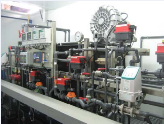
Pilot plant Membrane Bioreactor (MBR)
