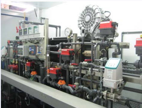
MBR pilot plant
